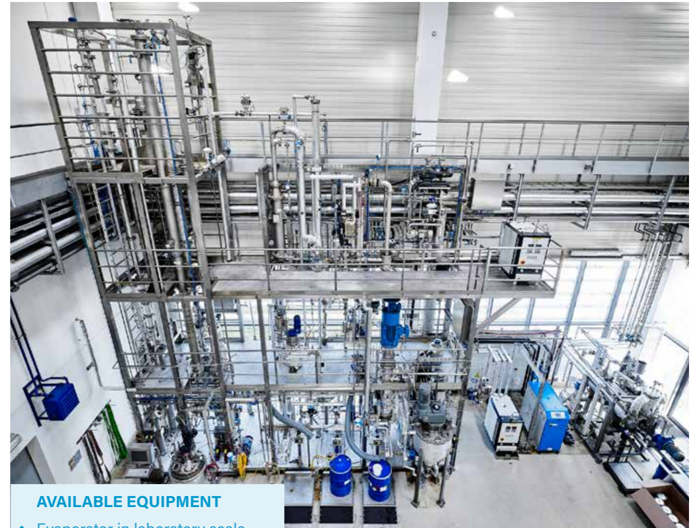
State-of-the-art equipment for testing and R&D. © GIG Karasek
